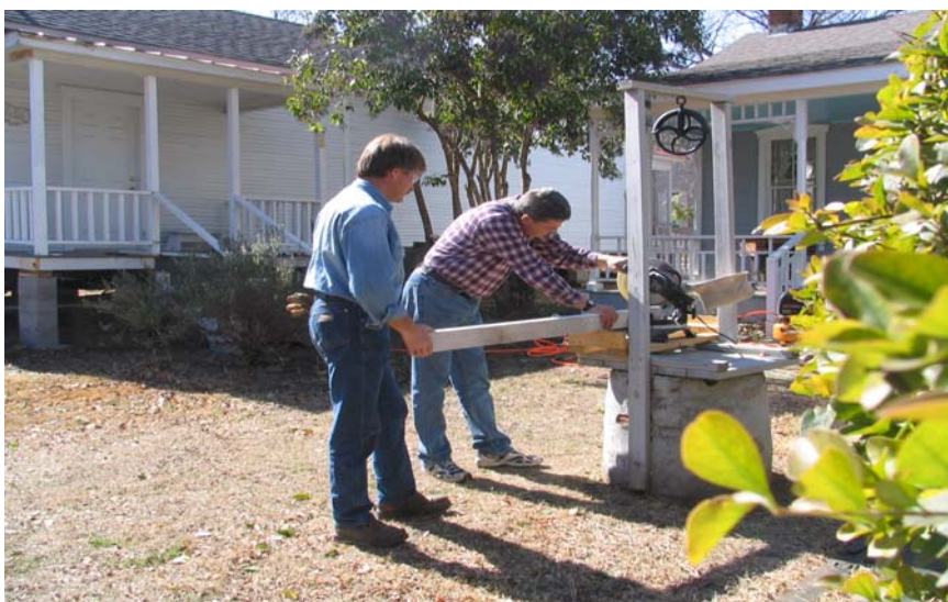
Front Porch Friday volunteers work on the Dixie Store in preparation for the grand opening and ribbon cutting on May 7. Volunteer projects don't always require tools! Call to find out more!
